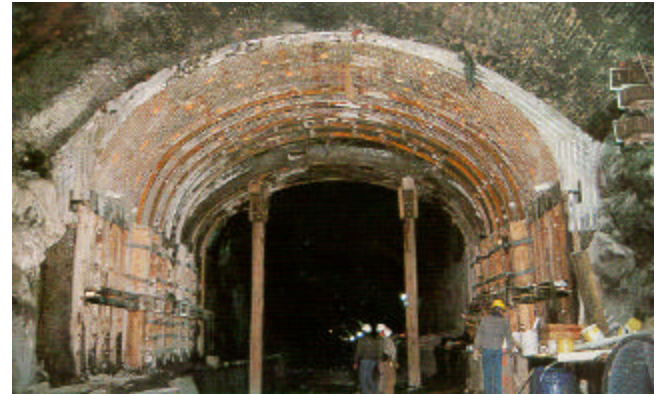
At left is the installation of temporary supports. At right, the installation of the new liner.
