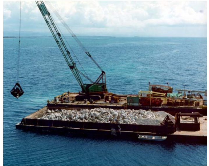
The ocean platform and installation procedures utilized in the implementation of MRCE's geotechnical design for the 3.5 mile outfall included extensive scour backfill for protection of the piping.
