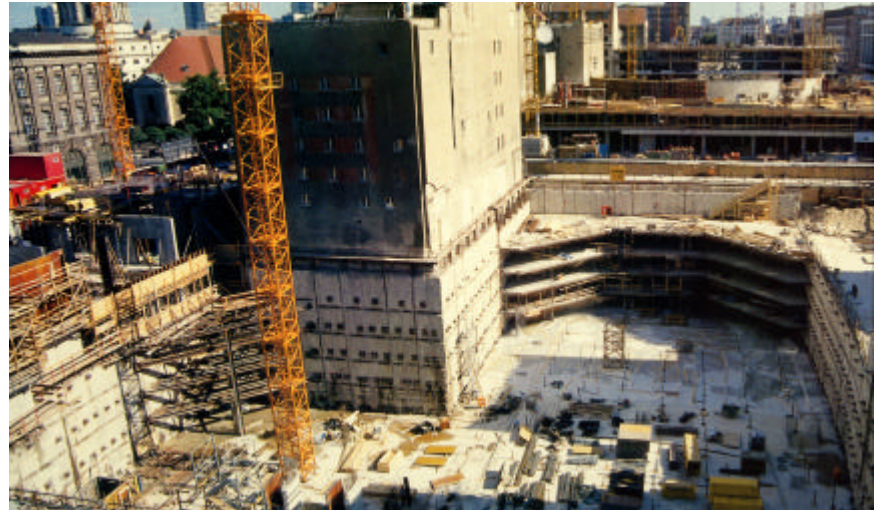
Construction proceeding for the five level deep below-grade parking garage beneath a hotel.
