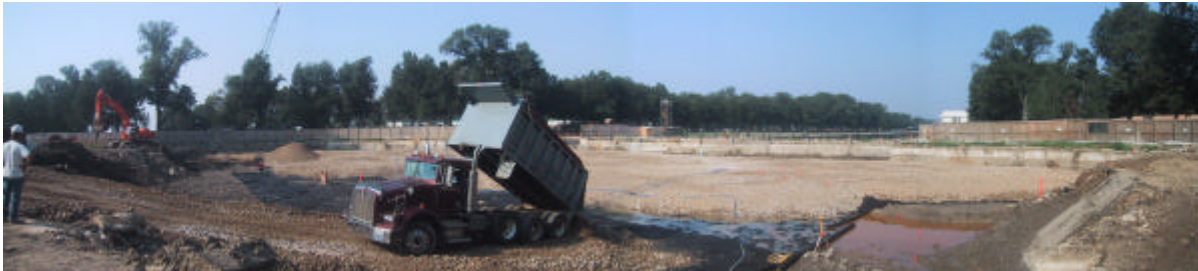
Above left: Site photo taken mid-February 2002 showing the concrete slurry wall under construction. The ceremonial elm trees being protected are outside the slurry wall. Lower left: Site work photo taken 7/16/02. Above right: Artist's rendering is an aerial view of the completed Memorial.
