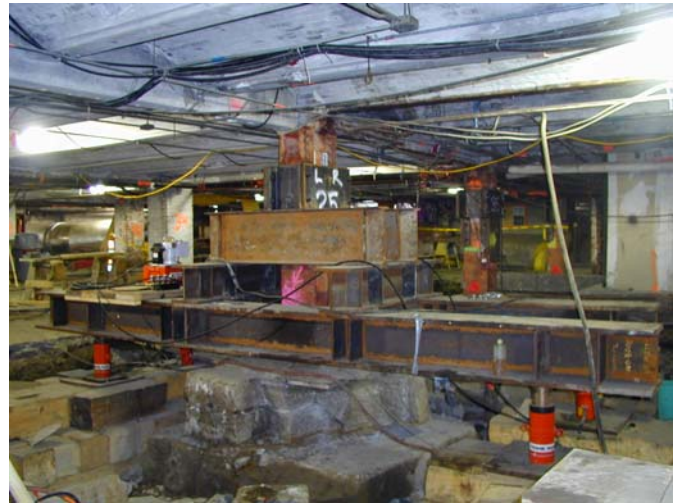
The Russia Wharf Complex (above left) is comprised of historic buildings in a waterfront area of Boston. The graphic shows how the tunnel was constructed below the buildings, which were occupied during construction. Above is the underpinning system in August 2000.
