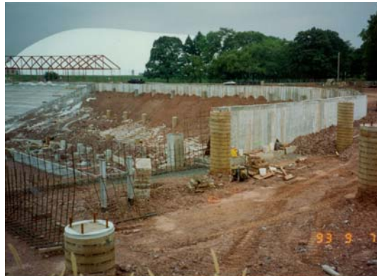
Photos taken during MRCE's investigation show the displaced retaining walls.
