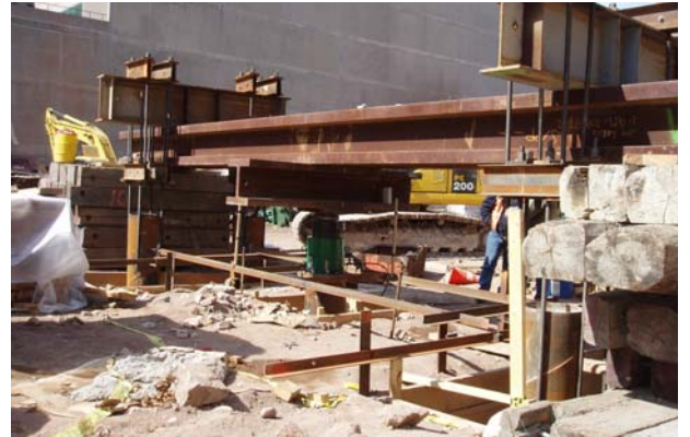
Upper right: Excavation at 270 Greenwich. Lower right: Conducting pile load test. Above: The building in relation to the WTC area construction. Center: Artist's rendering of the new building.
