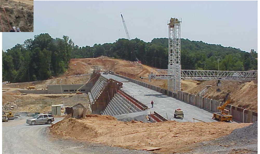
Construction photos taken in April 2002 (above) and June 2002 (at right) show progress of RCC dam and earth embankments.
