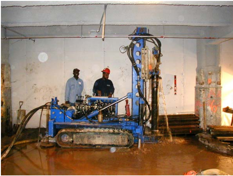
Above: Installing mini-piles under low headroom using reverse rotary drilling rig. The rig requires only 9.5 feet of headroom. At right: 4 foot lengths of drill casing enable drilling under low headroom.
